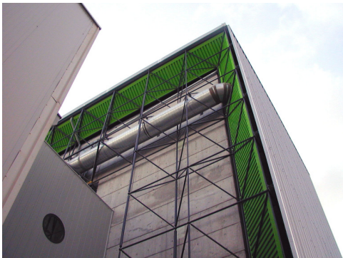
KBA Press Extension , HaAretz Press Facility, Tel Yitzhak, Israel Completed 2002
