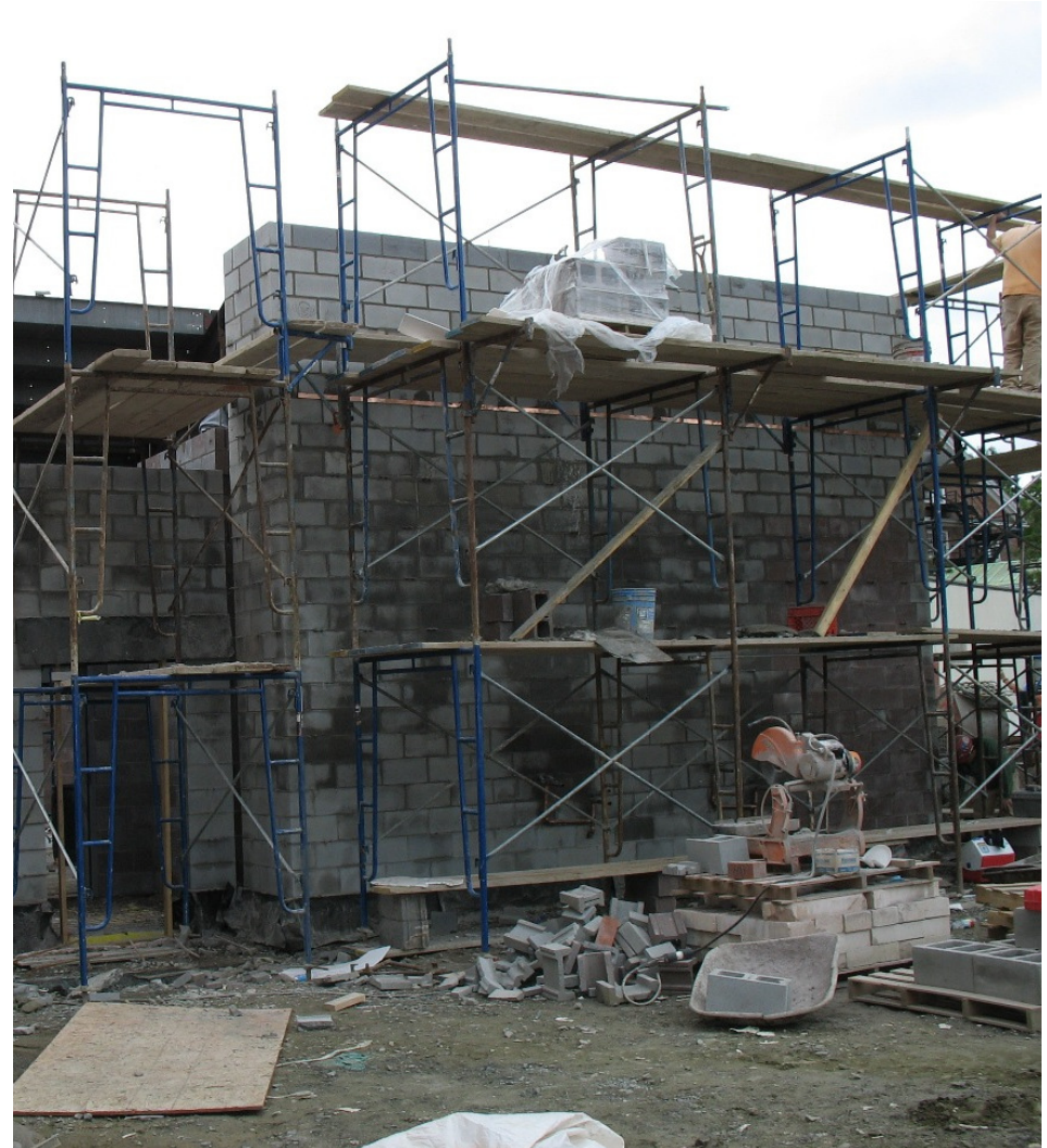
Fire-rated Masonry Enclosure
